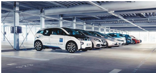
Electric charging station: Employees in Ditzingen have access to 86 charge points in the company’s own parking garage. TRUMPF is also electrifying its vehicle fleet.
