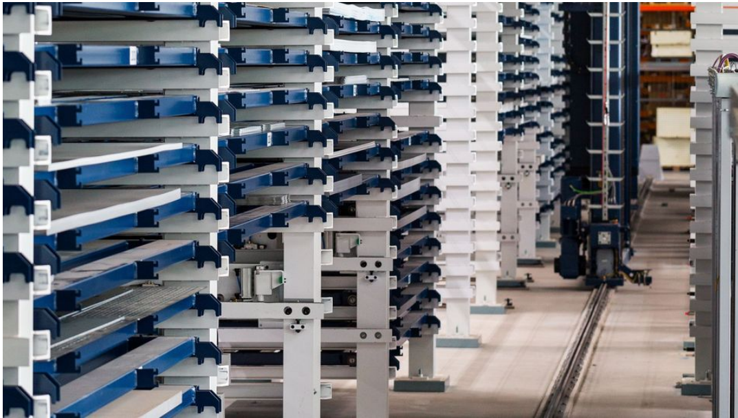
The storage system has 582 storage bays for large-format metal sheets. © Thomas Abe
