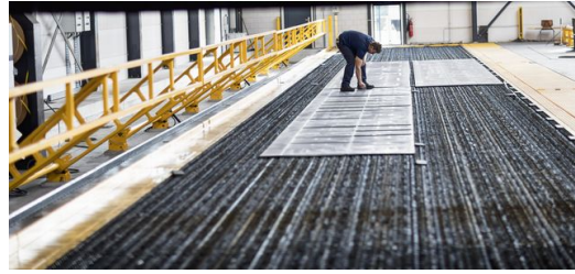
Because the table of the laser machine is at ground level inserting sheets is easy (Photos: Norbert Voskens).
