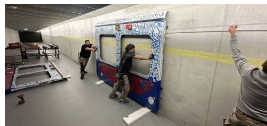
The subway train art was put in place using brackets produced in-house on a TruMatic 7000.
