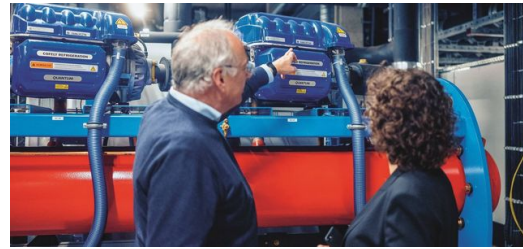
Blueprint: The right combination of heating and cooling applications can reduce energy use.
