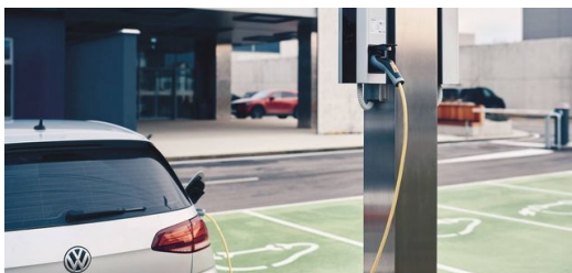
<p>Sustainable development – the charging stations for the company's vehicle fleet are powered by rooftop solar panels.</p>
