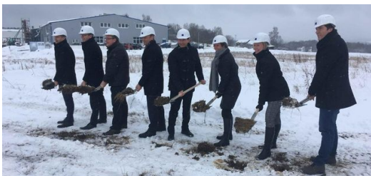
The ground-breaking ceremony for the new production hall at the TRUMPF site in Hettingen in January 2019. 120 employees are to move into the competence center in two years.
