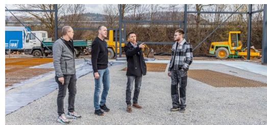
DELO is planning on relocating to neighboring Hechingen in September 2023. Construction work is in full swing. With a developed area of 2,000
